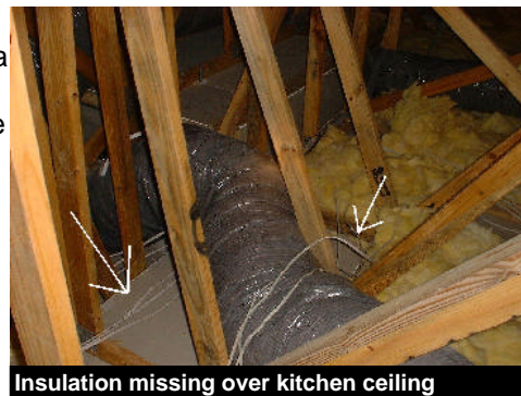
Insulation missing over kitchen ceiling
