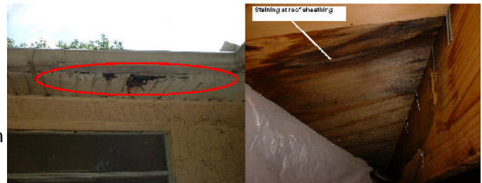
Damaged Overhang/Roof Problems/Leakage
