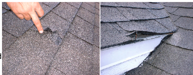
Protruding staple - Uplifted edge flashing
